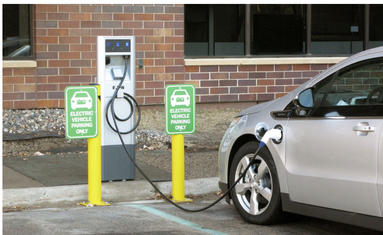
Expanding access to electric vehicle charging stations will help create an EV-ready community.
