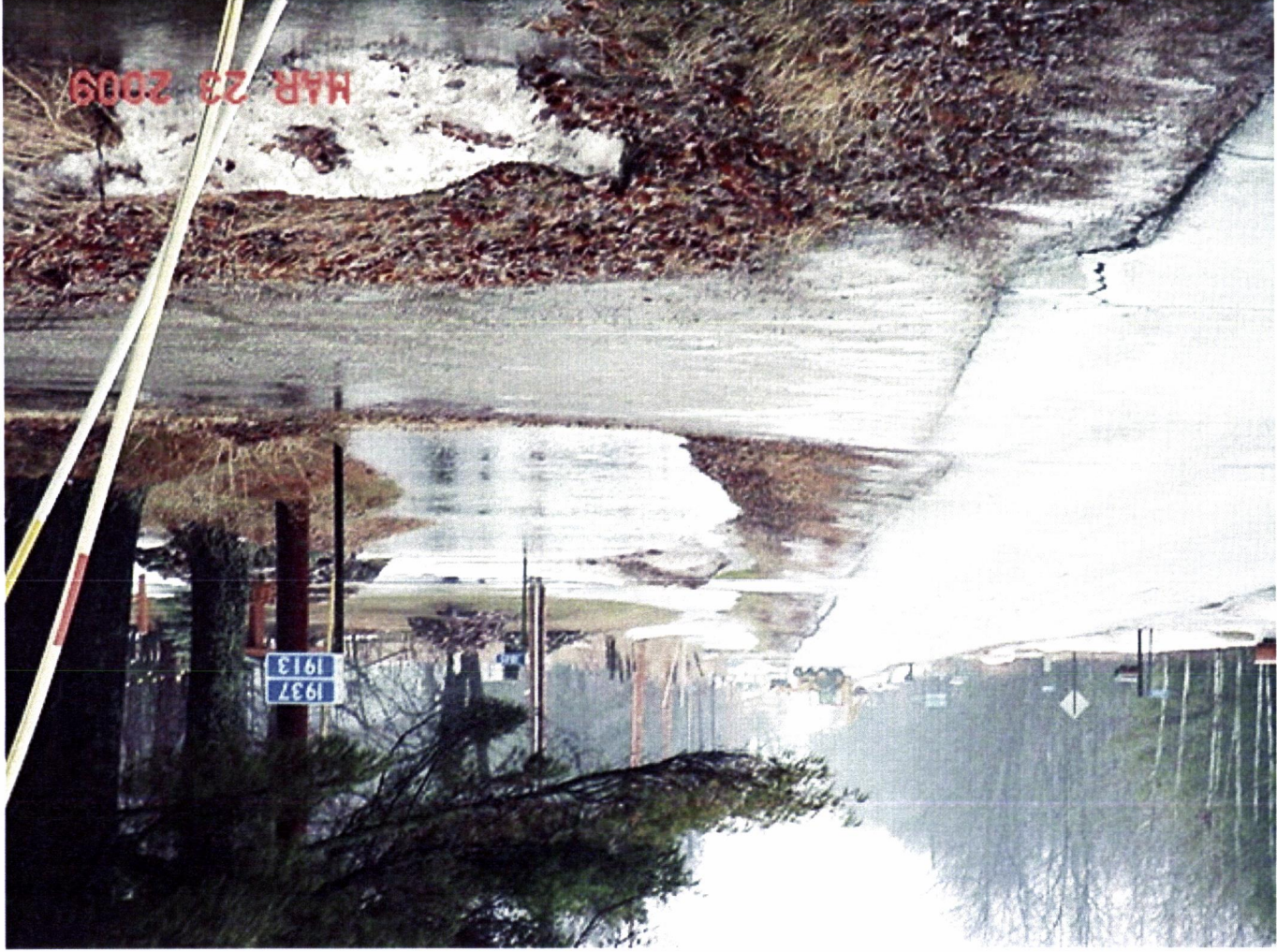
Drainage Issues - Islevievw
