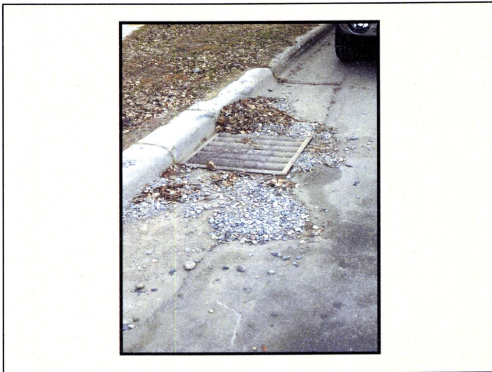
Stormwater Utility Catchbasin with Debris from Area Construction Project.
