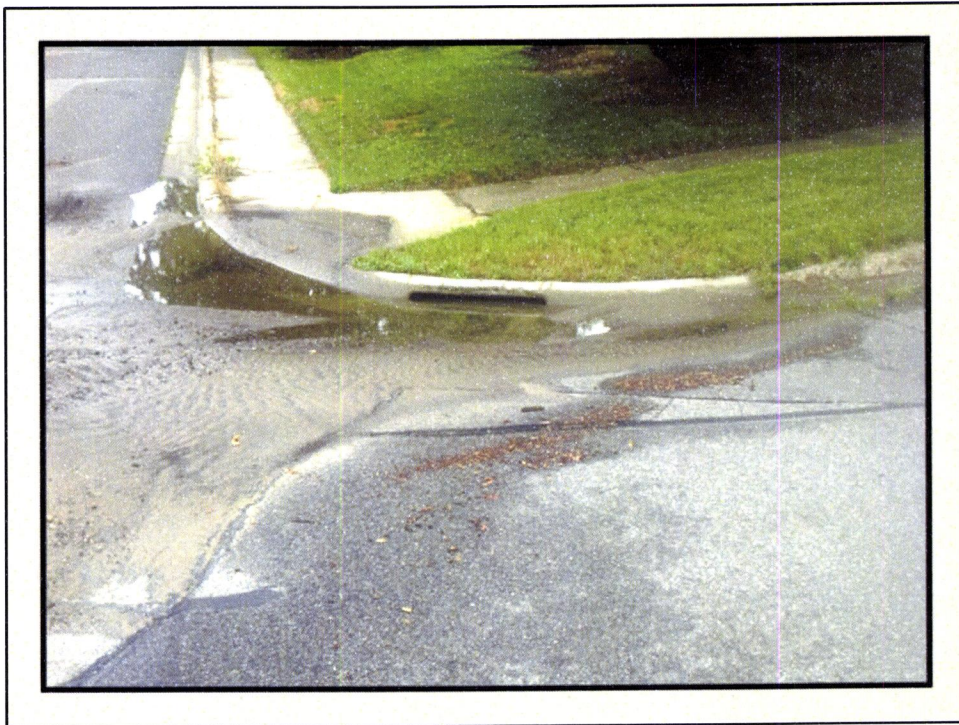
Alley Washout Plugs Stormwater Utility Catchbasin
