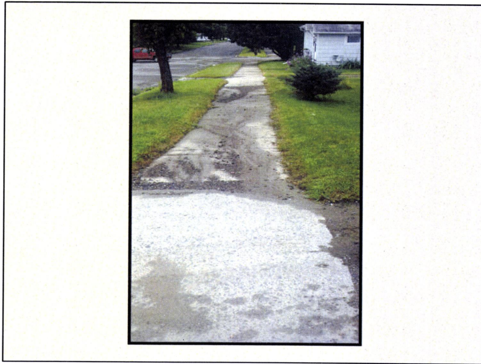
Alley Washed Out onto Sidewalk
