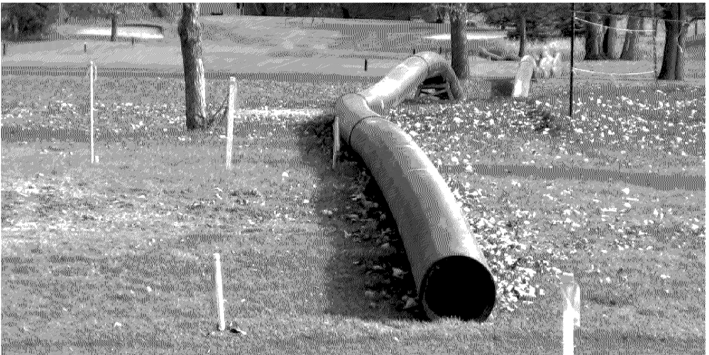
Roughly 12,000 linear feet of forcemain connects the two communities and transfers wastewater across the Minnesota-North Dakota border, under the Red River of the North.
